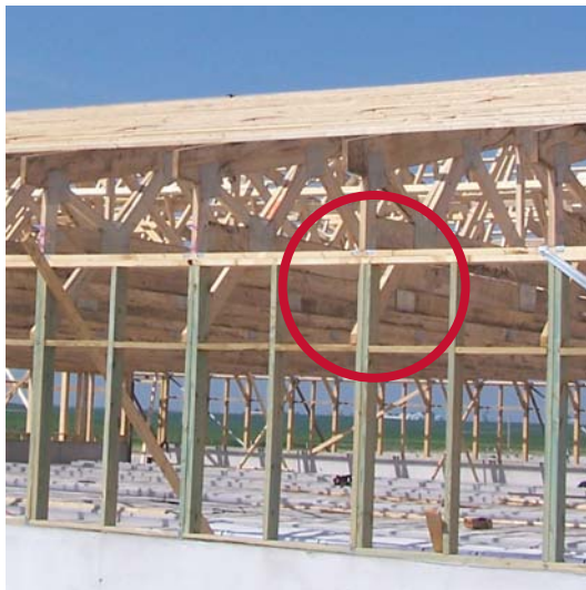
Figure 1. Knee brace used on an agricultural building.
